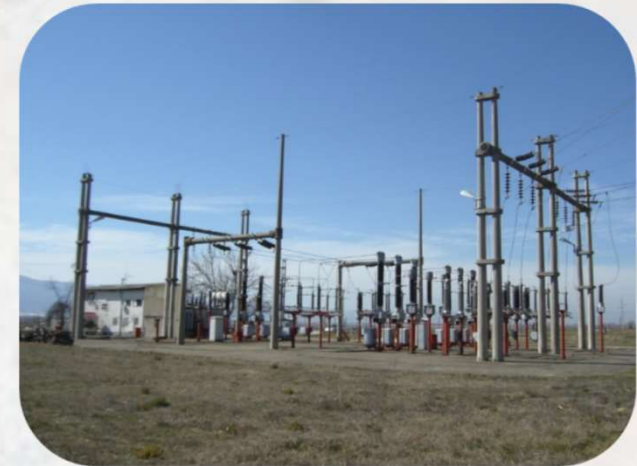
Existing MEPSO 110kV Substation Sushica
